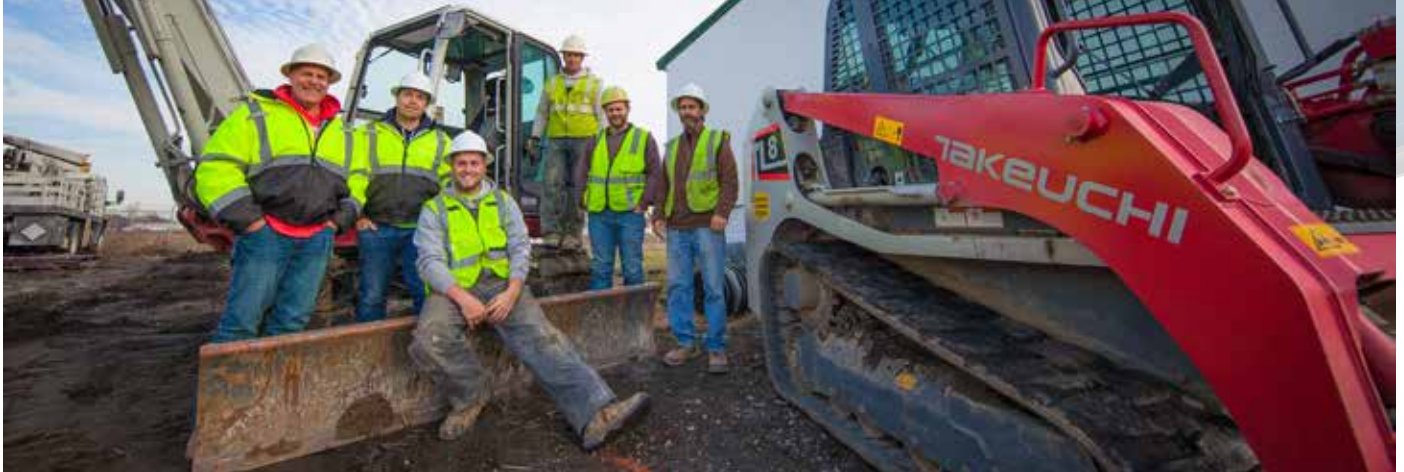
Kinnison's crew has been very satisfied with its Takeuchi equipment. The combination of dependable equipment with the crew's expertise and experience is a winning combination. (Left to right:) President Dave Kinnison, Operator Dylan Kinnison, Pipe Layer Andrew Bockrath, Pipe Layer Ben Linebagh, Foreman/Operator Chris Waddle and Operator Rodney Pettit.
