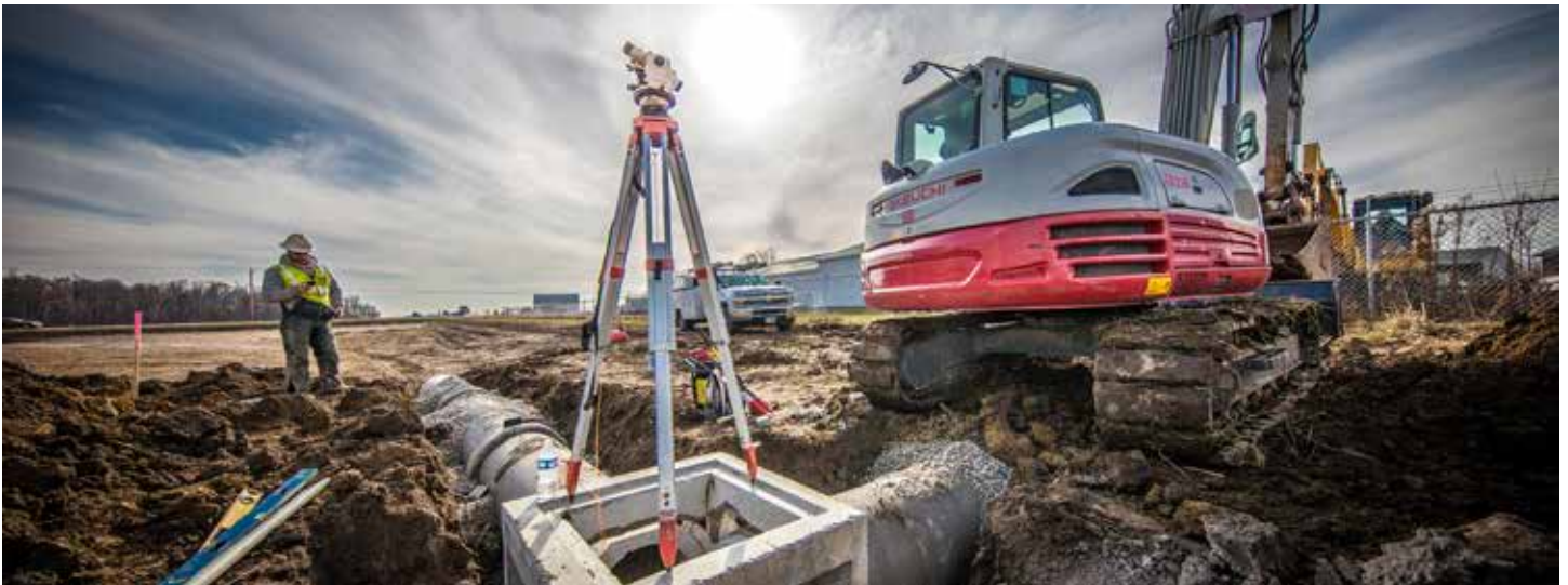
Kinnison Excavating pipe layer, Ben Linebagh, onsite in Piqua, Ohio with the company's Takeuchi TB290 excavator. The Skinner Painting project involved moving 5,000 yds. of dirt, building a detention basin and nine building pads, and installing 1,500 ft. of 12" and 18" storm sewer.
