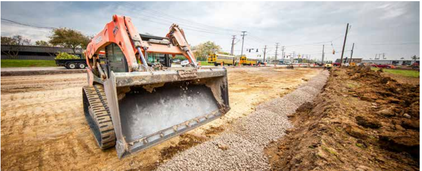
Miller Bros. Kubota SVL95-2S Operator Taylor Blausey works on the company's Shier Rings Road/University Blvd. project in Dublin, OH. The comprehensive 1.1-mile reconstruction and realignment includes paving, traffic signal and street lighting, water main, sidewalk, sanitary storm and sewer and electrical duct bank work.
