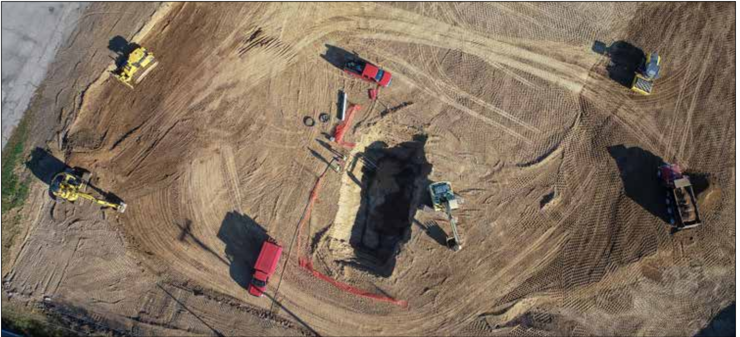
Completion of storm sewer, sanitary sewer and water work on the 4.6-acre site was performed in an impressive 90 days, assisted by a Komatsu D61PXi iMC dozer (top left).
