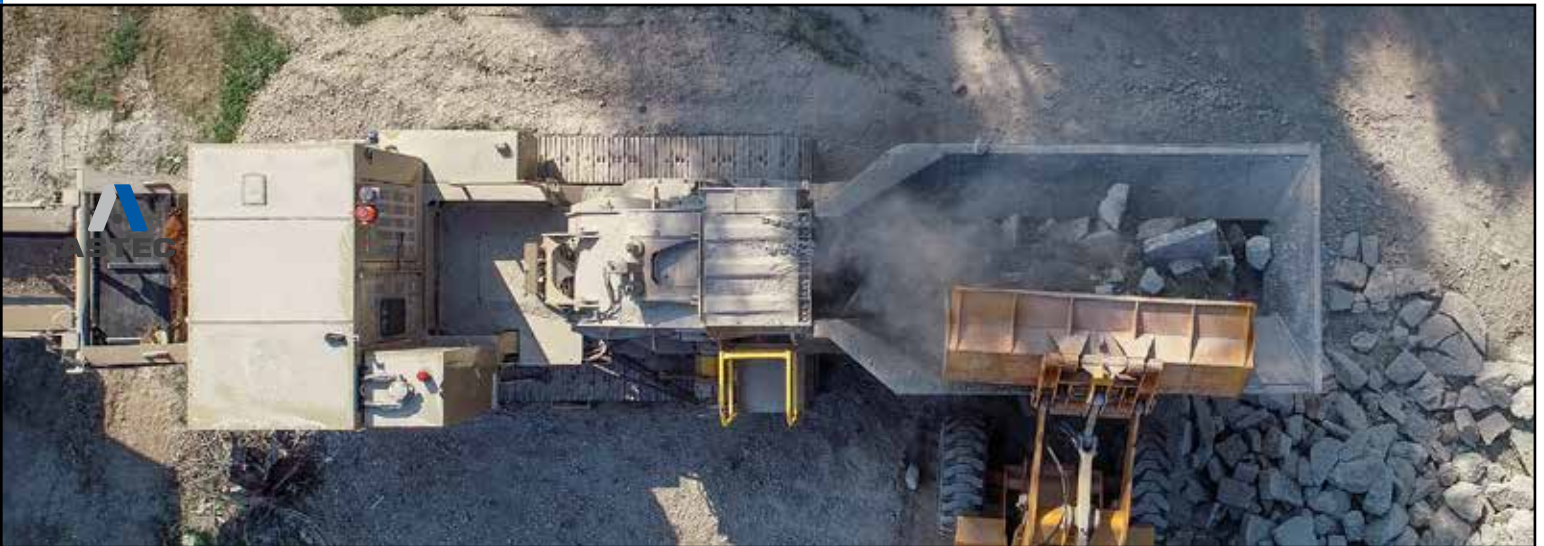
Balsbaugh Excavating's Astec GT440 crushes up to 300 tons of concrete per hour onsite, just outside Englewood, Ohio.
