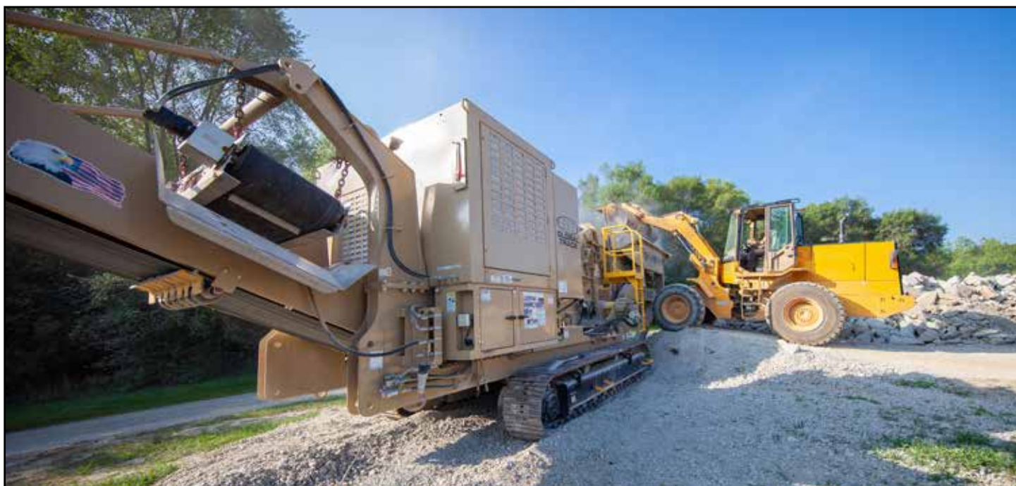
Operator Randy Bowman—a 36-year veteran—loads concrete into a GT440 producing 411/304 sand, as well as 57 and 2 products.
