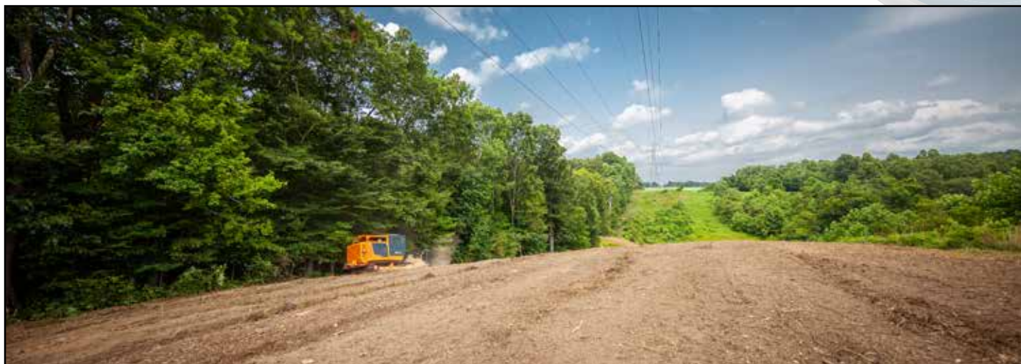
Jerrod Watts has an entire career of land clearing experience. Watts is pictured above in a CMI C400 clearing for a 12-mile, 138 kV transmission line rebuild just outside Philo, Ohio.
