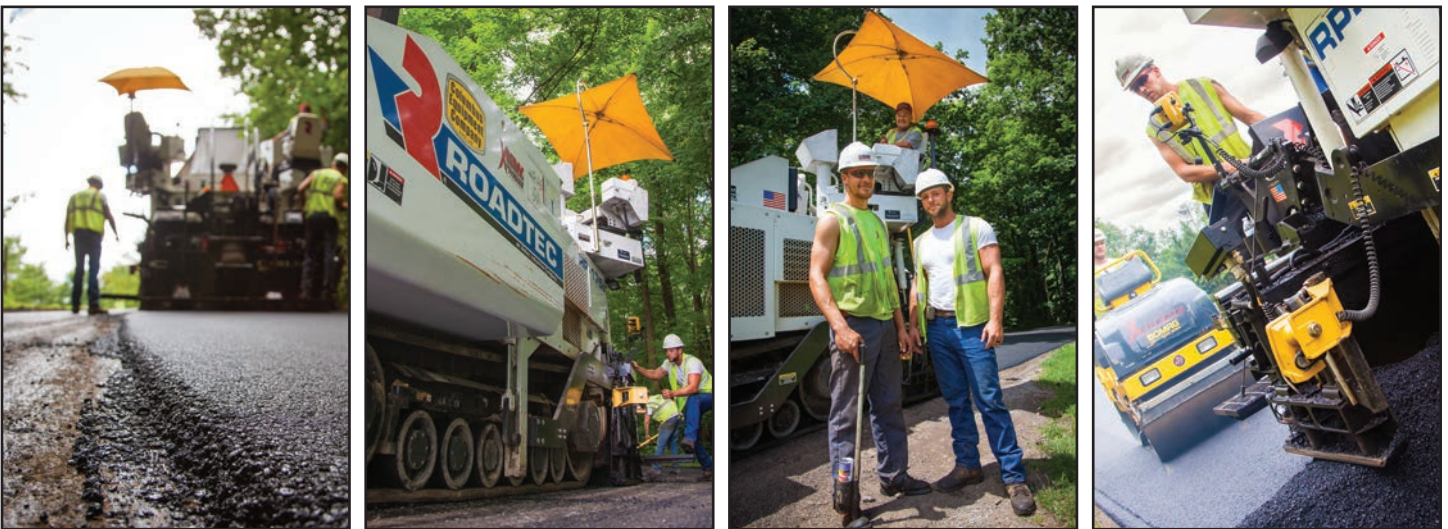
(Left) Consistent, high-quality mat. (Second left) The RP-175e is highly maneuverable due to the unit’s rubber track system. (Second right) Law General Contracting-Xtreme Asphalt’s Foreman Scott Vierstra, Operator Paul Roux and Screwguy Tom Finlay. (Right) Scott Vierstra and Rollerman Chris Robison work on Sunset Hill, on the Denison University campus in Licking County.
