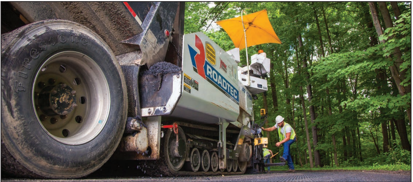
Law General Contracting-Xtreme Asphalt's Roadtec RP-175e paver has enabled the company to expand the paving services it offers. Pictured above on a 500-ton, two-day project at Denison University in Tree City USA Granville, OH, the RP-175e is known for being mechanically simple, technologically advanced, and easy to operate.
