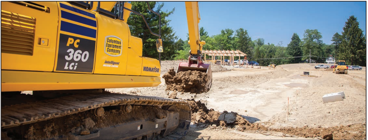
The company's Komatsu PC360LCi showed its prowess on the Geauga Park District, 74-acre Hyde Kaplan Park project. Operator Mike Lewis estimated a 25-30% time savings on the project, including the creation of five bioretention swales (pictured).
