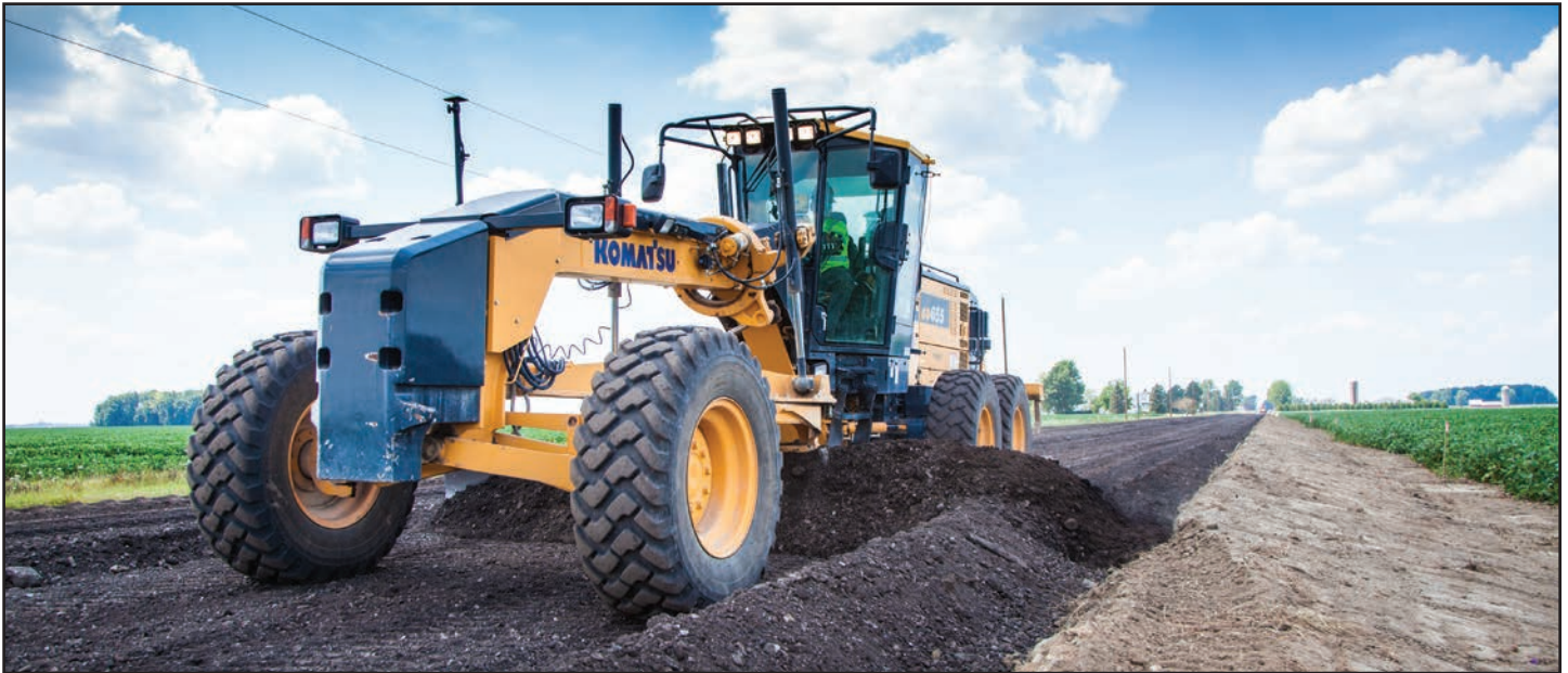
A Komatsu GD655 grader works Weston Road between Thompson and Crockett on the $4.35-million project, which included 9.7 miles of roadway reconstruction and 23,000 tons of HMA placement.
