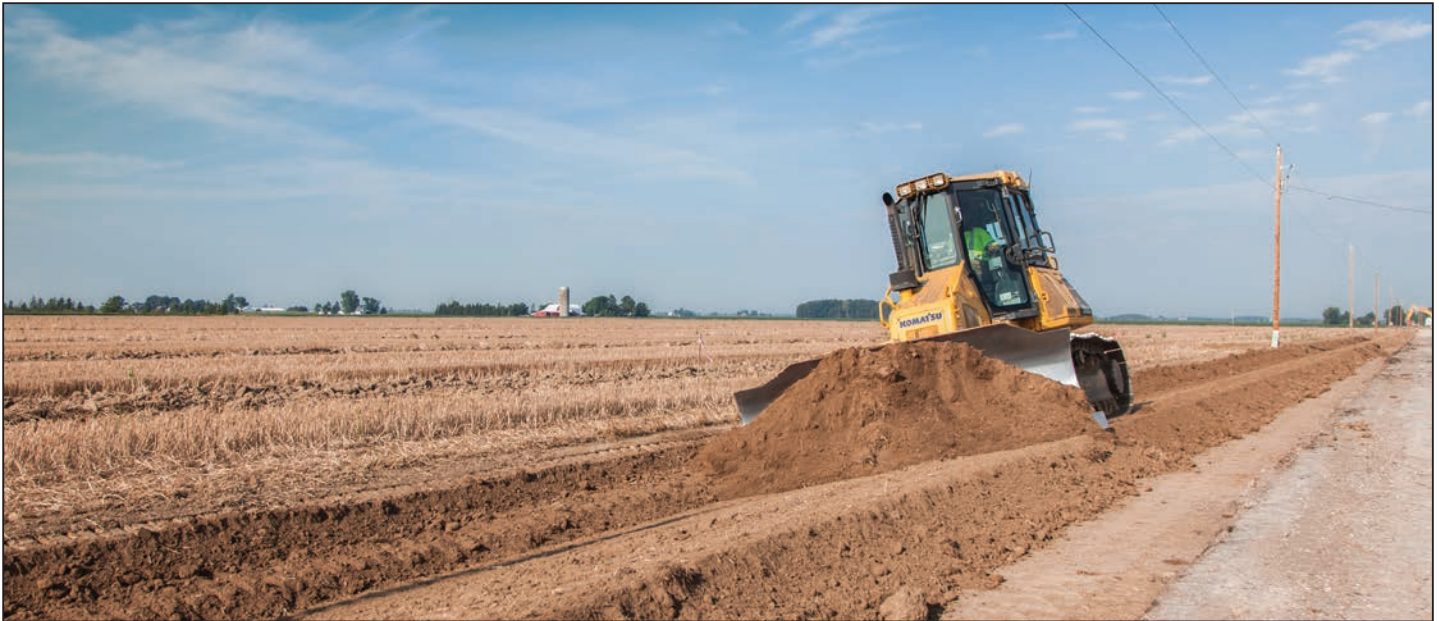
APC's Operator Toby Kolinski (above and lower left) puts the company's Komatsu D51EXi's power, control and visibility to work cutting slopes and ditches. iMC accuracy can reap significant rewards when removing 30,000 cu. yds. of dirt and placing over 17,000 tons of aggregate.
