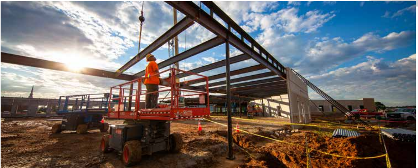
Link-Belt RTC-8065 SII Operator Jacob Darby sets structural steel in the early morning hours on the Genesis Coshocton Medical Center site. Work on the project—involving 60,000 sq.ft. of space and 250 tons of steel—will take place over 16 months.
