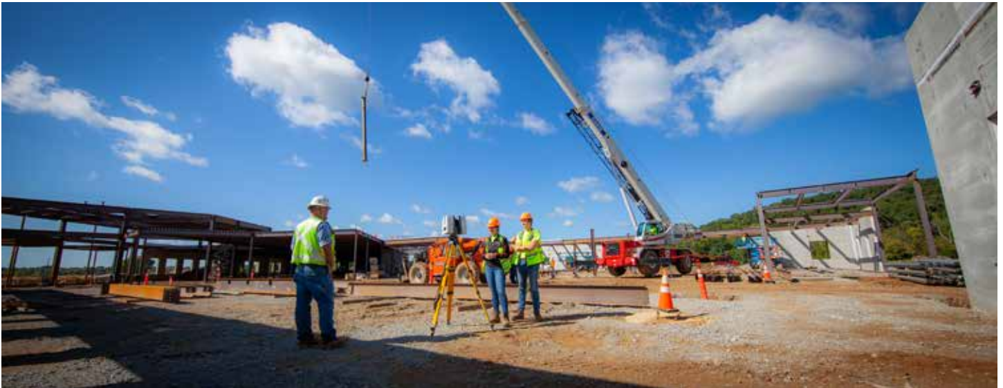
Danis Surveyor Doug Frye (left), accompanied by University of Cincinnati coops Erica Horschler and Blake Reinstedler, with a Leica P40. The state-of-the-art laser scanner can perform one million measurements per second, formatting the data into a 3D point cloud, enabling crews to achieve a high degree of accuracy and efficiency.
